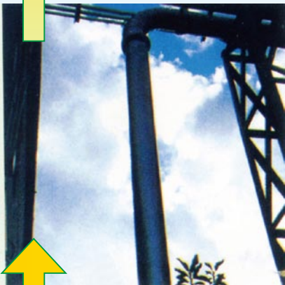
▲ 垂直約5M送進乾燥機 Push into dryer over about 5 meters
