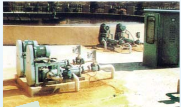
▲ 餘剩污泥抽吸Pump Pump for dirty mud suction
