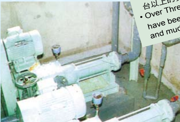
▲ 下水、生屎尿輸送Pump Pump for underground Water and shit transport
